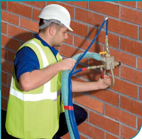
EcoBead installed externally
